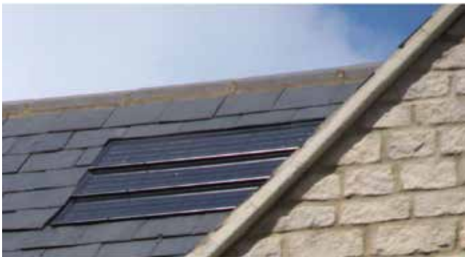
Integrated photovoltaic panels
