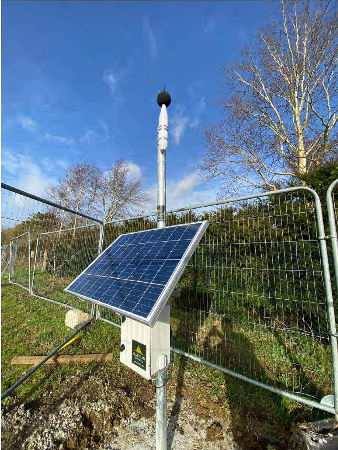
Figure 2.2: Automated Monitoring Equipment Installed at Position 1 (Position 2 Identical)
